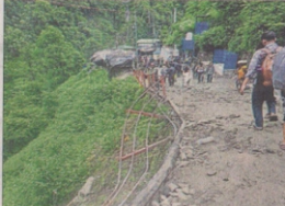
A slide-railing was damaged by boulders that rolled down from hills near Junglechauti on the Kedarnath route in Rudrapur district on Wednesday.
